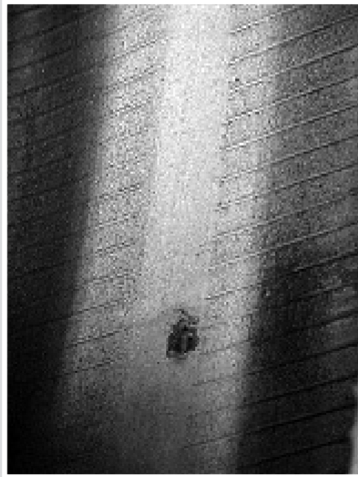
Puncture/penetration Inside View
